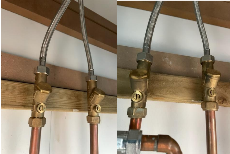
Example of Flexi-Hoses found on site.
